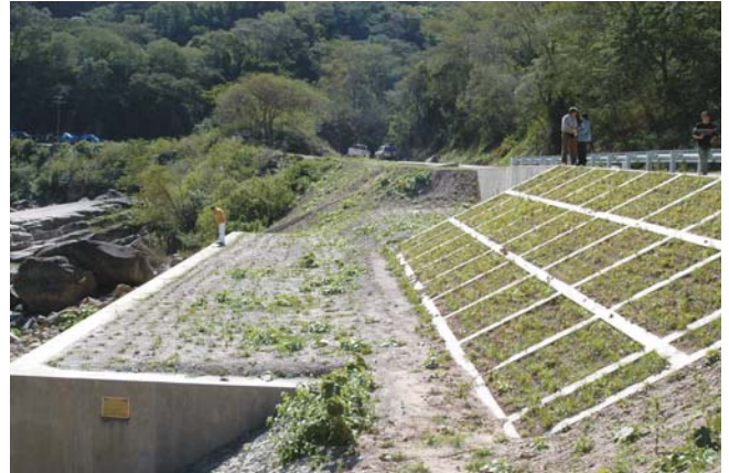
Road shoulder reinforcing by stepped structure and restorative planting (Photo: Fernando Xavier Cuellar Otero/JICA)
